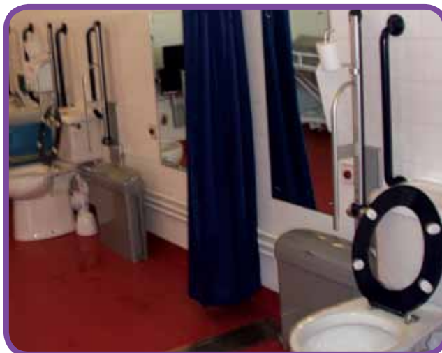
Keighley Leisure Centre's 23 sq m facilities are large enough to include two peninsular layout WCs with a privacy screen, enabling more efficient use by a visiting group
