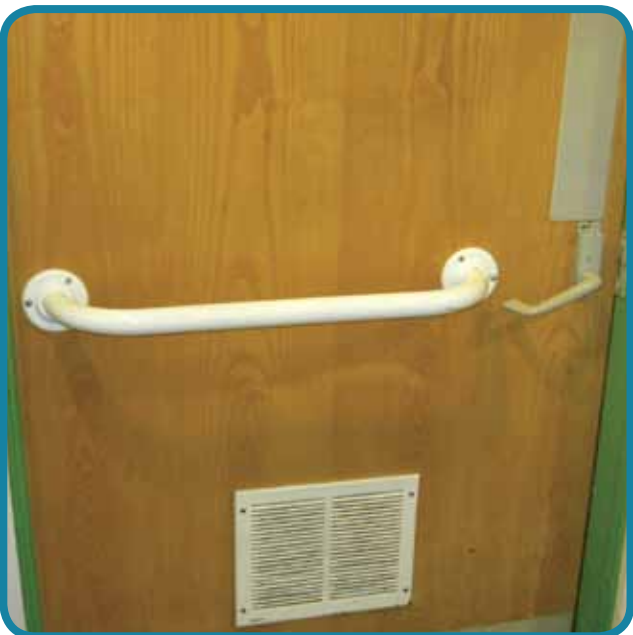
A light action lever lock on the inside of this toilet is easy to use and changes the occupied / vacant indicator on the outside
