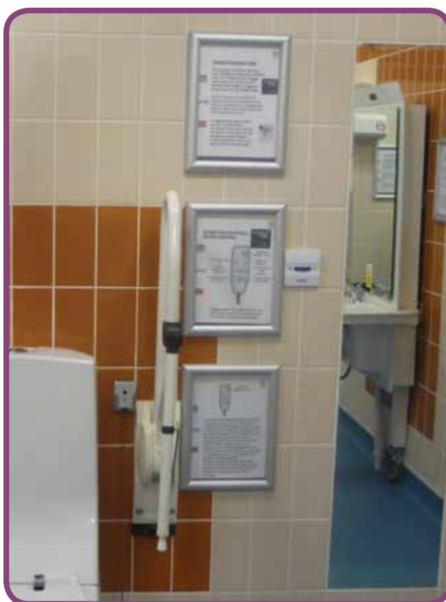
Information signs in the Tonbridge CP facility provide clear diagrams and instructions for using the equipment
