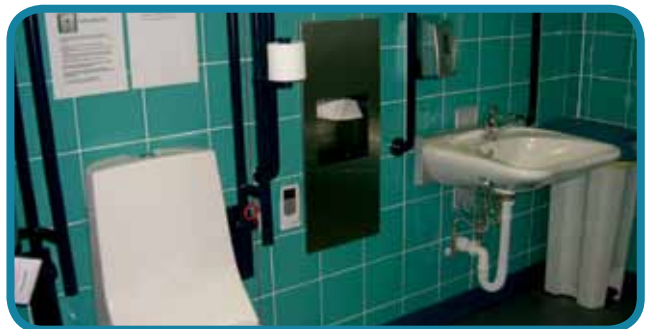
The fittings at the CP facility at City Hall, London, contrast visually with their background
