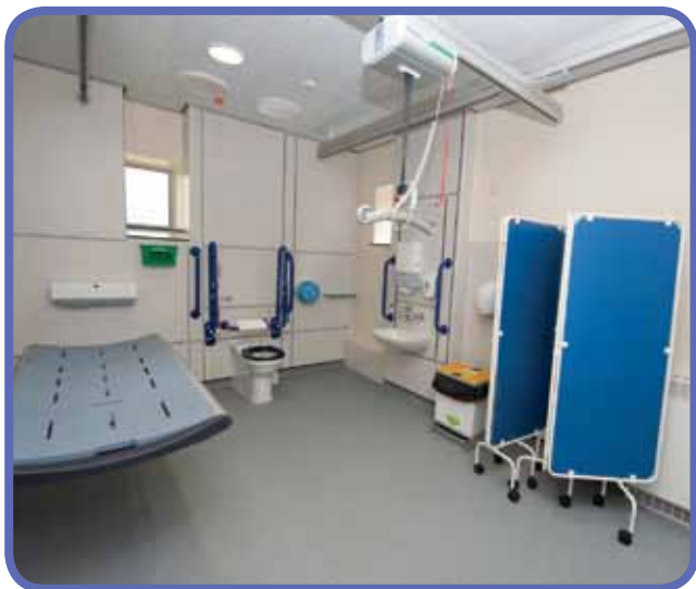
Changing Places facility for assisted use: minimum 3m by 4m in size, including a centrally located WC with space for assistants either side, adult-sized height-adjustable changing bench, a ceiling track hoist and privacy screen
